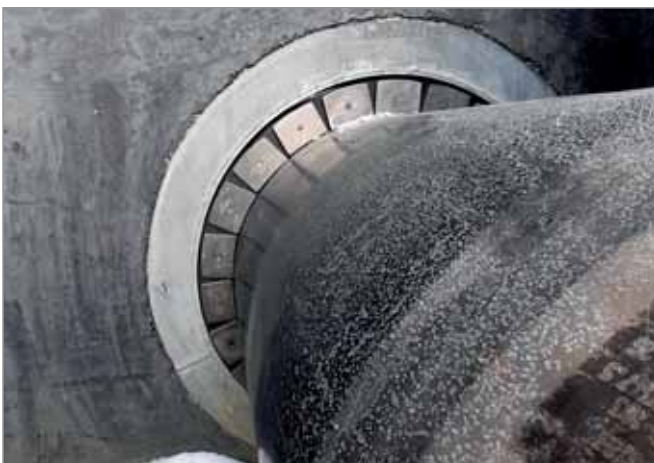
Sewer pipes 600 mm diameter
