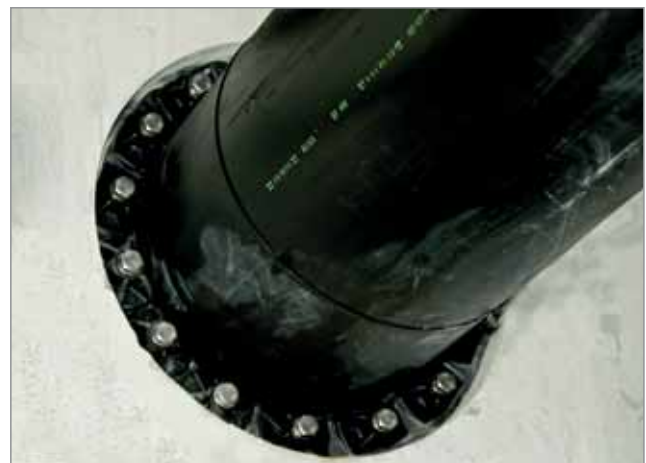
Water pipelines 250 mm diameter
